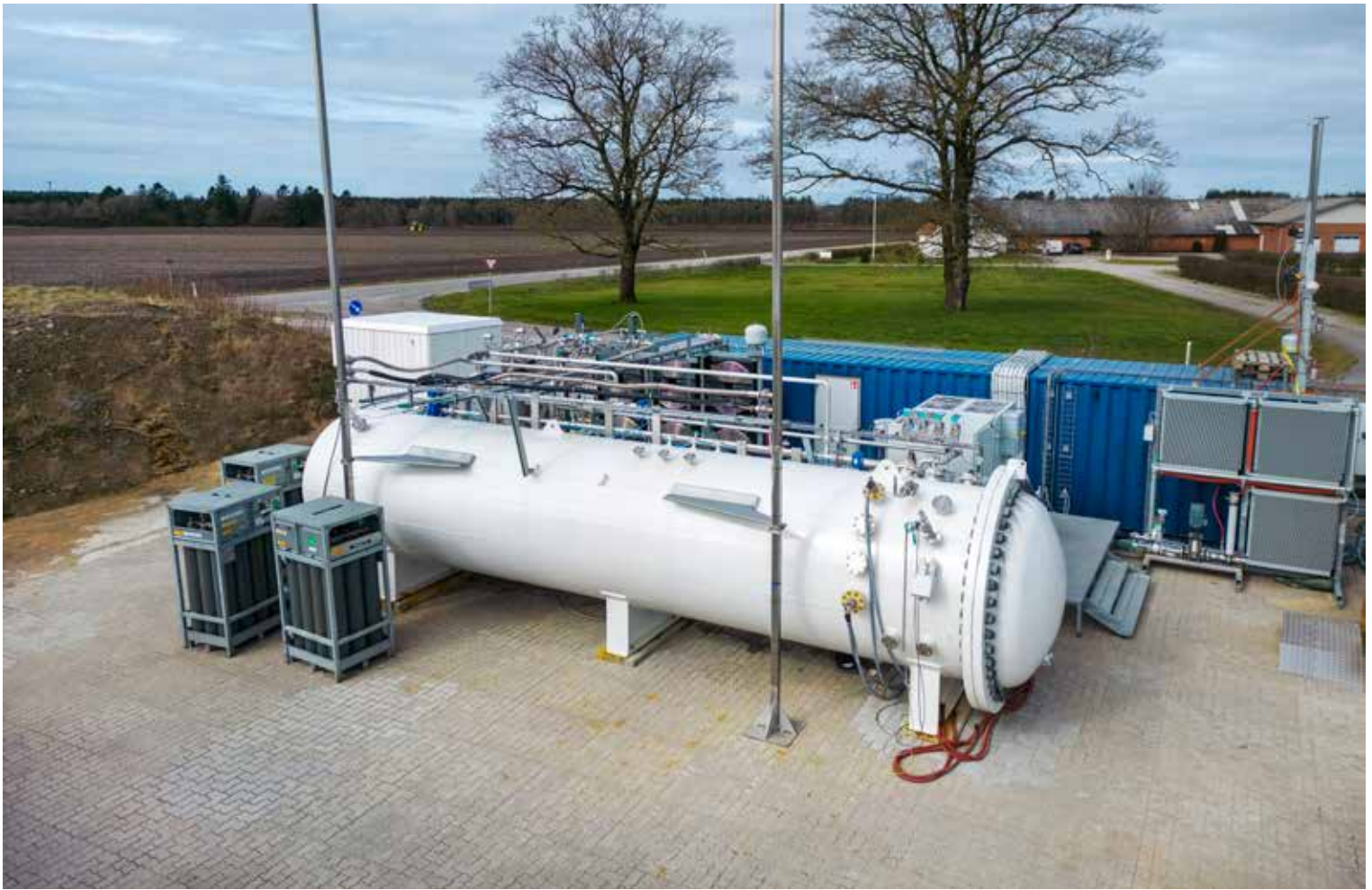
Revolutionary compact: The 3 MW HydroGen Electrolyzer integrated into a pressure vessel, resulting in an ultra-compact unit footprint. Depicted here at Stiesdal Hydrogen's test site in Give, Denmark.
