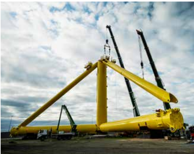
Quay-side installation with pin assembly of one of the three braces on the TetraSpar Demonstrator.
